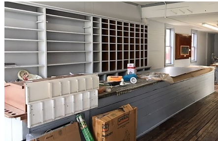
The front room at the Main Street site after it had its first coat of paint in many years
